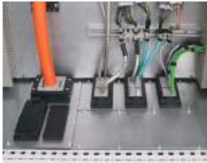
Cable routing via module plates in the base of a Rittal TS8 enclosure. Mounting with icotek gland plate KDR BMP.
