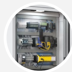
Control panel technology, DIN rail terminal blocks
